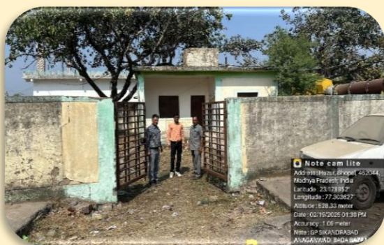
Sub Standard works of Anganwadi, Bada Bazar, Gram Panchayat Sikandrabad, Ratibad cluster, Bhopal
