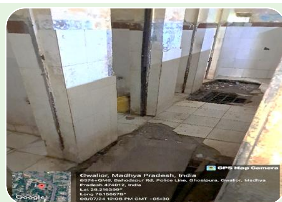
Photo-2.1.5: Dilapidated condition of washroom of male IPD ward in GMH Gwalior
