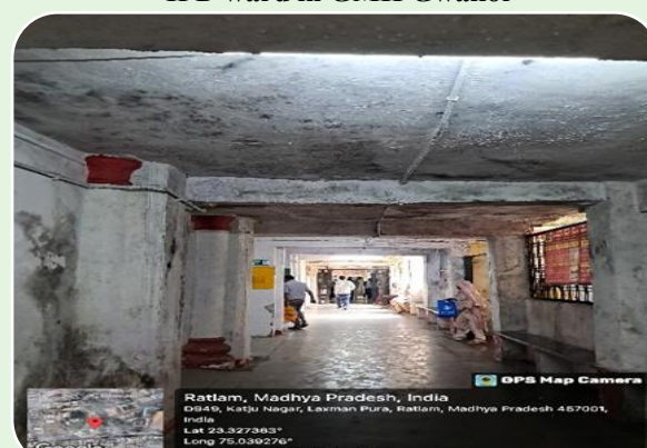
Photo-2.1.8: Dilapidated condition of hospital building of DH Ratlam
