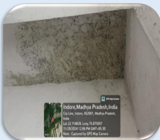
Picture-2.3: Seepage in ceiling of a room of Sakhi Niwas, KEH, Indore
