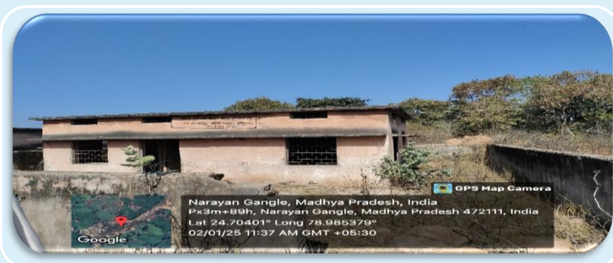
Photograph-1.5: Photo showing dilapidated condition of AWC in Dhimrola Narayanpur Village
