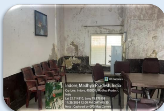
Picture-2.11: Seepage in dining area of KEH, Compound, Indore
