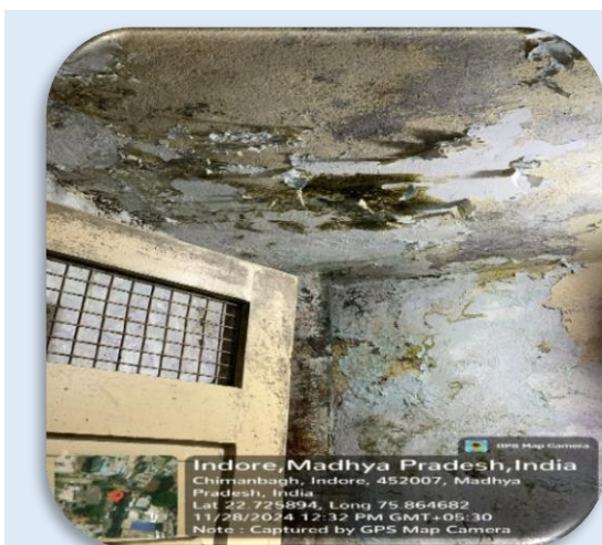
Picture-2.2: Damaged plaster and paint of AIMS WWH (Indore)
