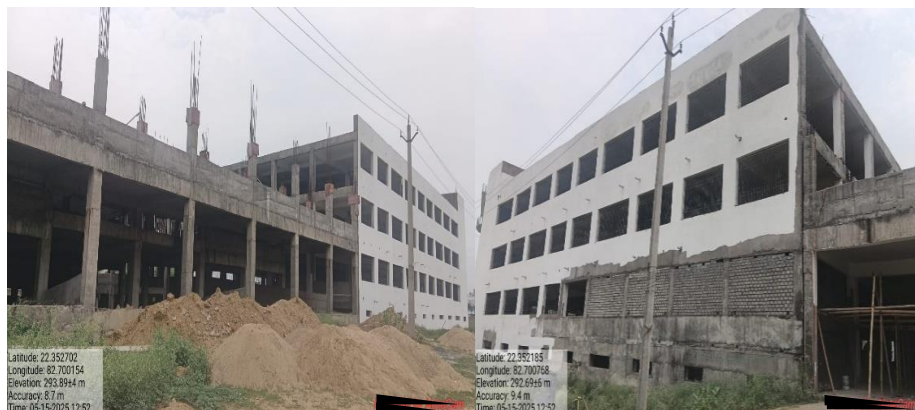
Picture 3.7: Photos of incomplete multilevel parking at Korba
