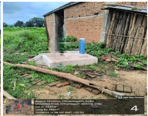
Photo 4.2: FHTC constructed, laying of distribution line not done and composite pipe lying open without connection (Kamardera habitation, Village-Bhithidih)
