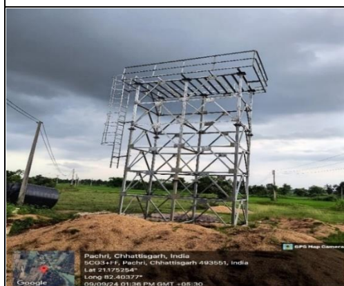
Photo 4.8: Incomplete OHT at Pandripani (Pachri), District: Mahasamund
