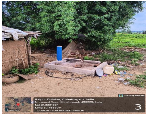
Photo 4.1: FHTC constructed, laying of distribution line not done and composite pipe lying open without connection (Kamardera habitation, Village-Bhithidih)
