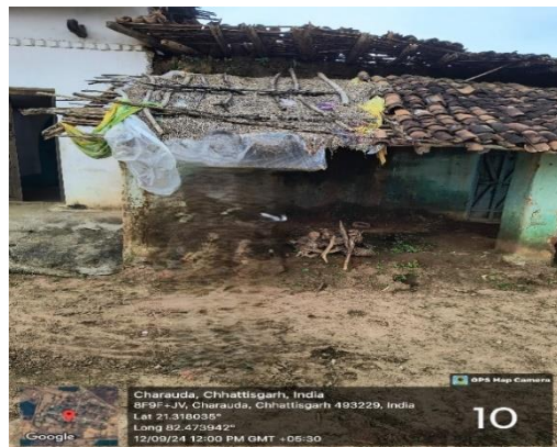
Photo 4.3: Distribution line did not reach and FHTC not constructed (Vidyanagar habitation, Village-Bhithidih)
