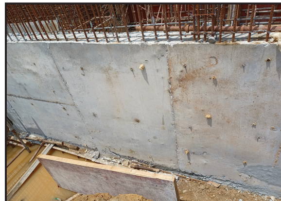
Picture 9D - Poor concreting in RCC wall construction at BIEC station
