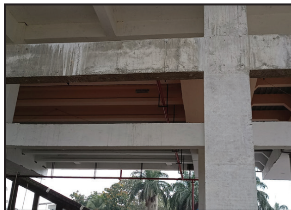
Picture 10B - Honeycombs in beams at Central Silk Board station construction
