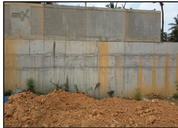
Picture 9B - Poor quality at Kothanur Depot
