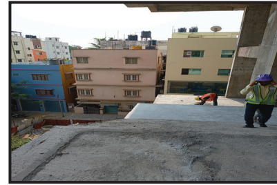
Picture 11A – Missing barricade and protection at staircase at Jayadeva Hospital station
