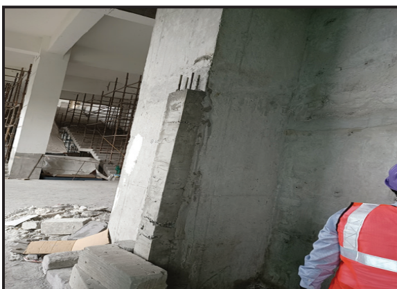
Picture 9E - Poor concreting in columns at Central Silk Board station
