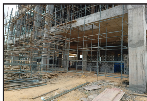
Picture 8B - Improper base of the formwork system and poor concreting at Kothanur Depot
