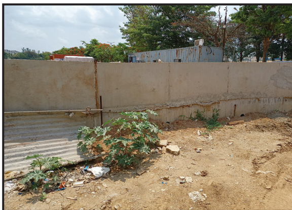
Picture 10A - Honeycombs and non-uniform concrete surface of retaining wall at BIEC station
