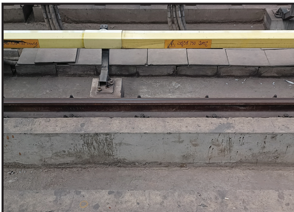
Picture 9C - Cracks on plinth beam below rails at Nagasandra Station
