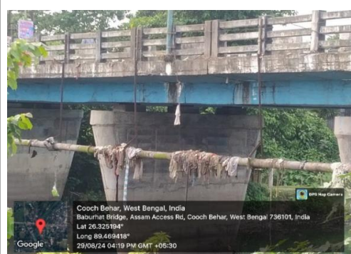
Figure 4.10: Pipeline hung with the railing of the Mora Torsha bridge at chainage 2.00 km of Coochbehar Dinhata Gitaldah Road under Cooch Behar Division (PWD)
