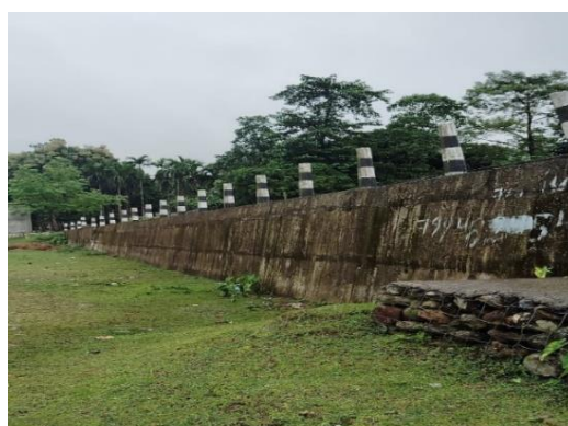
Figure 4.16: W type steel barriers not provided at 2.00 km of Coochbehar Sitalkuchi road over river Saltia
