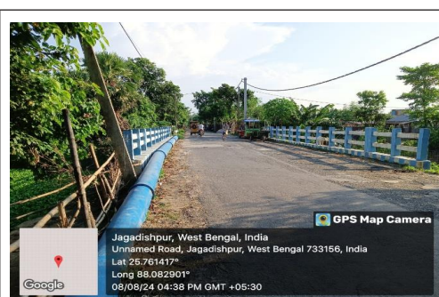
Figure 4.8: Pipe line laid on the superstructure of the Bridge at chainage 1.00 km of Makdampur-Bhatol Road under Uttar Dinajpur Highway Division PWD(R)
