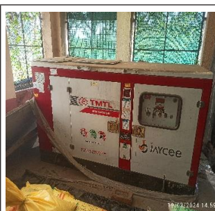
Figure 4.2: Generator set kept idle
