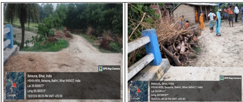
Image 4.1 and 4.2: Incomplete approach roads (both sides) of HLRCC bridge at Nonia Toli in Betauna Village under Patahi Block, Pakridayal (East Champaran)
