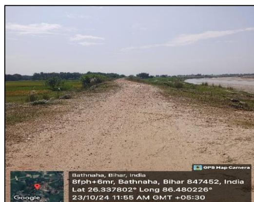
Image 3.1: Damaged GSB material on the top of the embankment
