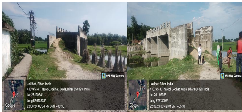
Image 4.3 and 4.4: Incomplete RCC bridge and its approach roads at Thapkol to Karhbana road near Thapkol village of Jokihat block (Araria)
