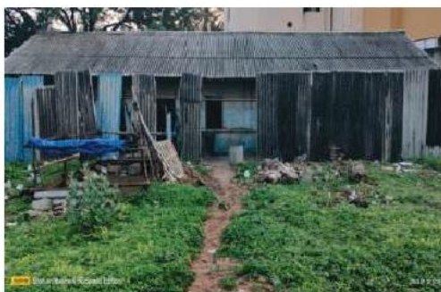
Picture 2.1: Existing building in dilapidated condition at Puducherry
