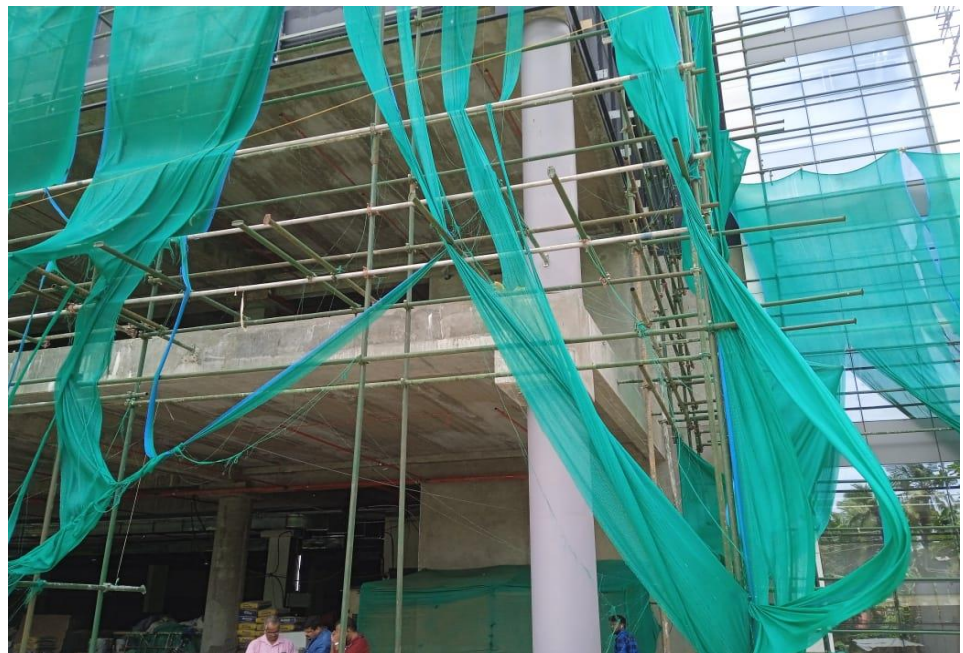
Figure 5.4 M/s Kalyan Silks building, Thodayad Junction, Kozhikode. Failure to provide quality safety net to prevent accidents. Photo taken by Audit party on 20 September 2023.
