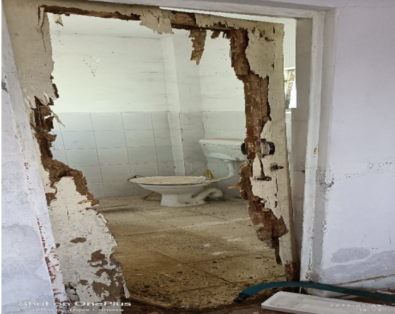
Broken washroom door in the residence of MOIC, CHC, Kotabagh, Nainital
