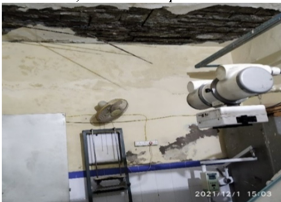
X-ray room in dilapidated condition at CHC, Doiwala, Dehradun
