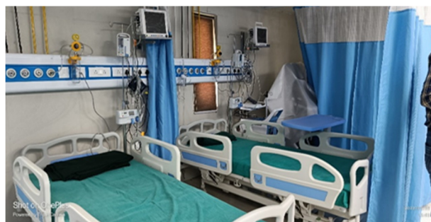
Photograph-: Non-functional ICU Ward in SDH Haldwani, Nainital
