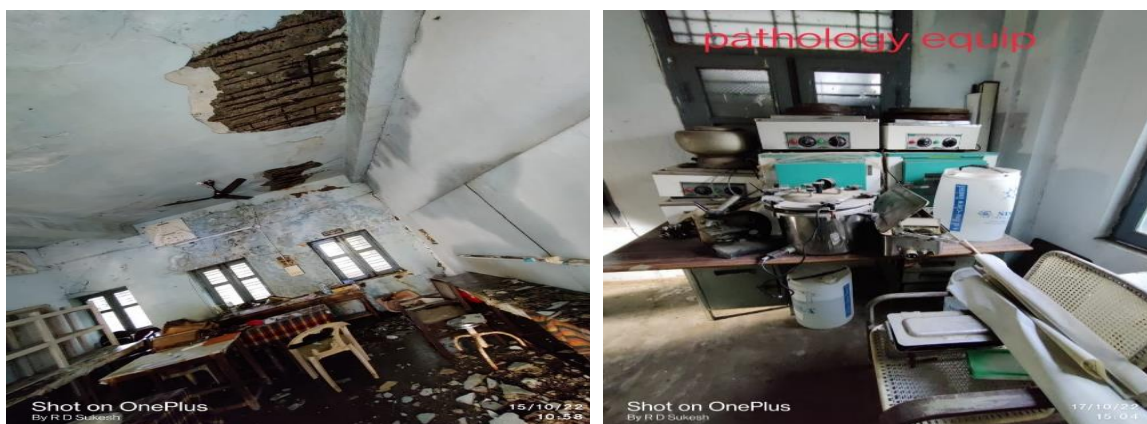
Figure 10.2: Dilapidated condition of Department of Pathology Block (October 2022)
