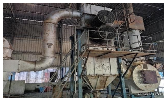
Incinerator in CBMWTF at Athivaram village
