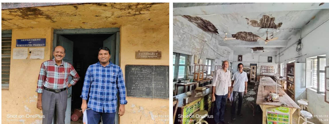
Figure 10.1: Dilapidated condition of Homoeopathic Pharmacy Block (October 2022)
