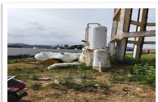
Figure 5.20 : Oxygen generator plant at AH Tekkali (June 2022)
