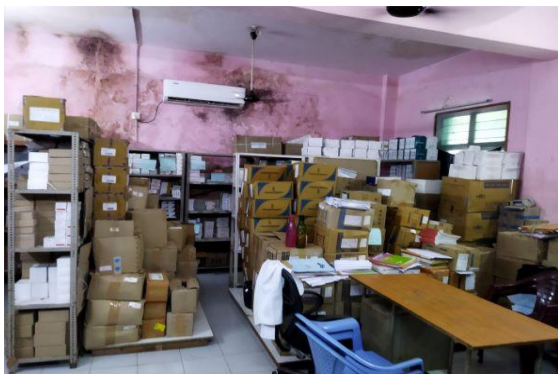
Figure 4.3: Seepage on walls in AH, Seethampeta (June 2022)
