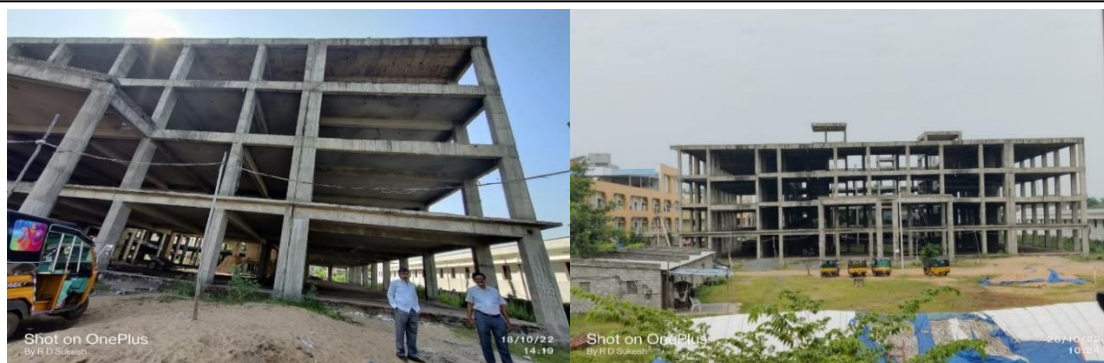
Figure 10.5: Incomplete structure of new building for Homoeo Medical College attached Hospital at Gudivada (October 2022)
