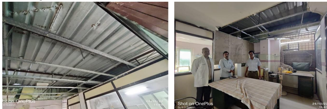
Figure 10.6: Condition of Ceiling in Outpatient Departments of Dr. Gururaju Govt. Homoeo College, Gudivada (October 2022)
