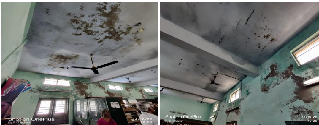
Figure 10.4: Dilapidated condition of Library Building of Dr. Gururaju Homoeo Co, Gudivada (October 2022)
