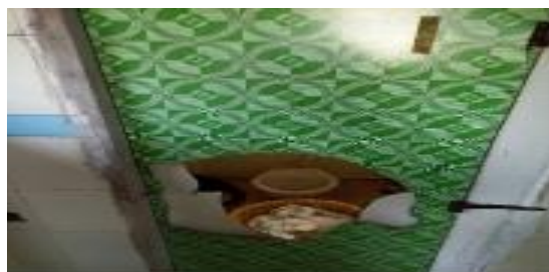
Figure 5.14: Dysfunctional Toilet in Girls Hostel, GMC, Srikakulam (June 2022)
