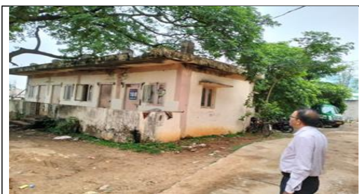
Figure 7.1: BWH at Seethampeta in Dilapidated condition (June 2022)
