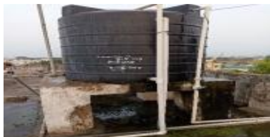
Figure 5.13: Overhead tank leakage in girls' hostel, GMC, Srikakulam (June 2022)
