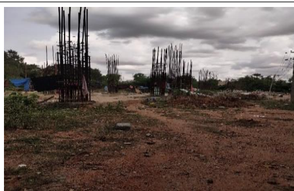
Figure 3.3: Abandoned work of burns ward at GGH, Anantapur (September 2022)
