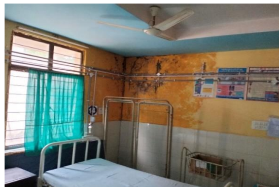
Figure 5.7: Seepage in ward at AH Seethampeta (June 2022)
