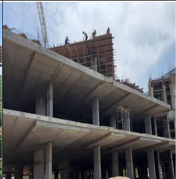
(4) Workers engaged without safety net and wearing safety belt in construction of high rise building at The Landmark, Indore
