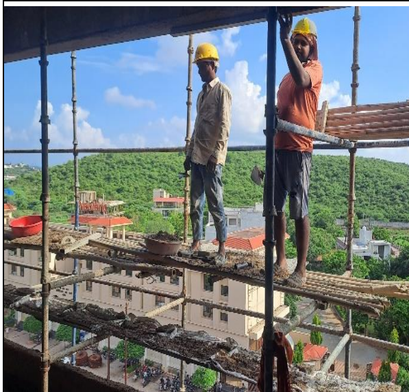
(3) Workers engaged without safety net and wearing safety belt in construction of high rise building at One Business Centre, Gwalior
