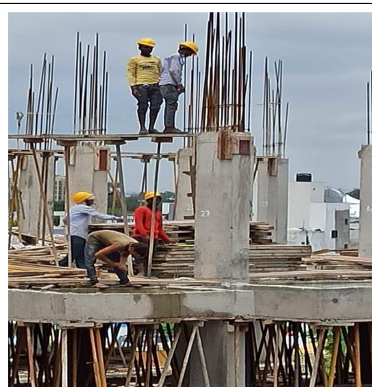
(2) Workers engaged without safety net and wearing safety belt in construction of high rise building at M/s Virasha Nisarga, Bhopal
