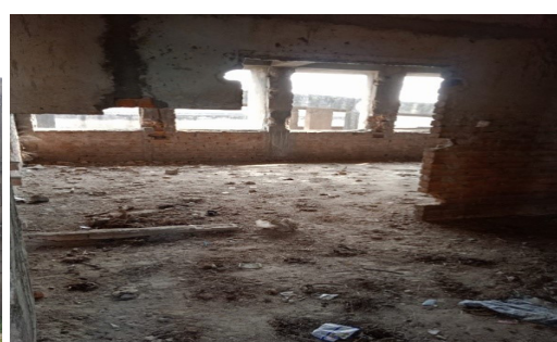
Image 2: Damaged walls and windows (due to lack of maintenance)
