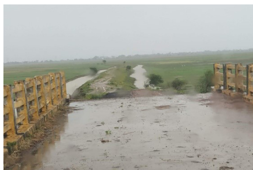
Image 3: One side of the bridge (Kumhra side) remained unconnected (as of 30.09.2021), with the 3 km length of road, having been constructed on other side of the HLB (Laxmipur side)
