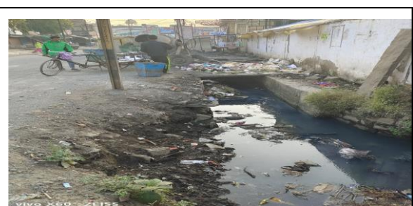
Image 2.39: Dumping of waste in drains
