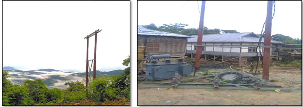
Incomplete works certified as completed at Rovakot Village, Churachandpur District.
