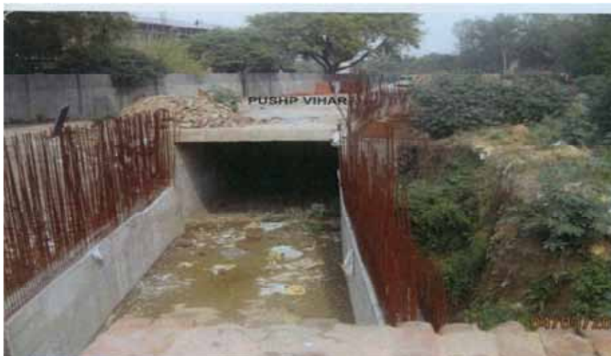
Abandoned work of covering of PushpViharNallah
