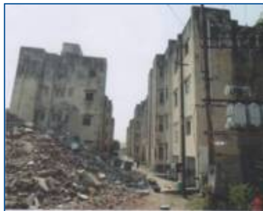
Picture 4: Collapsed EWS housing complex at Madhavnagar (obtained from the records)
