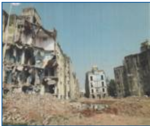
Picture 3: Collapsed EWS housing complex at Madhavnagar (obtained from the records)
