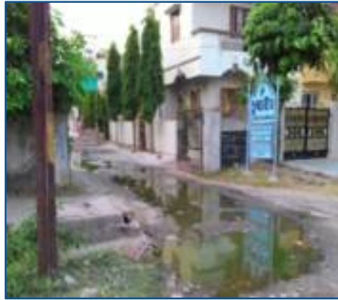
Picture 1: Sewage water accumulated in the Entrance of Krishnadeep Tenaments (02.06.2015)
