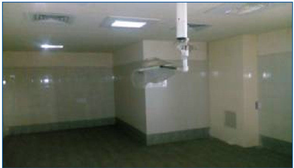
Picture 14: Non-operational OT at CH Surat (25.07.2015)
