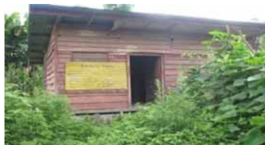
Picture-17: Poor condition of Labour Room of Maram Khullen PHSC, Senapati District Manipur
