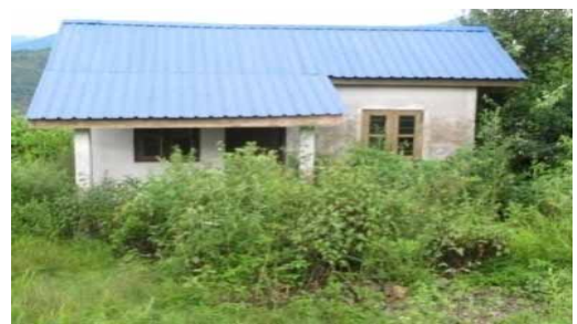
Picture-15: Unoccupied staff quarter surrounded by bushes at Maram PHC, Senapati District, Manipur
