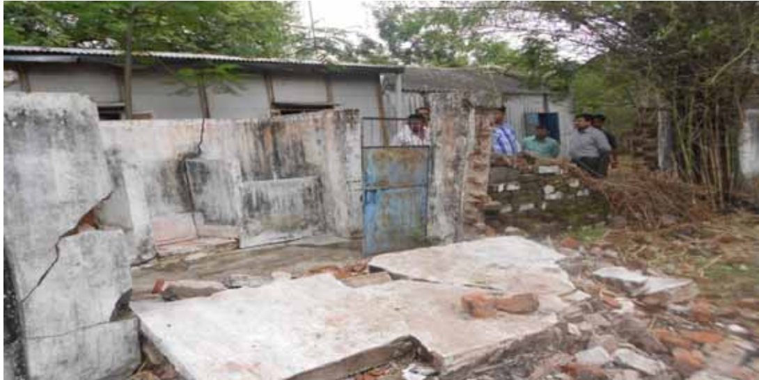
Picture-5: Damaged compound wall and girls' toilet of Primary School, Chandpuri Faliya, Dantol, Panchmahal, Gujarat
