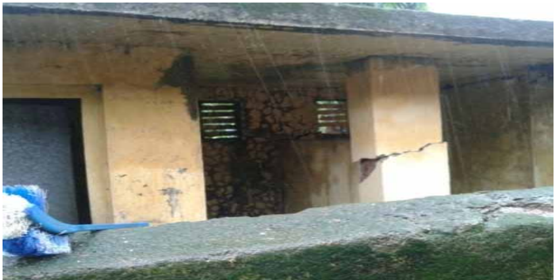
Picture-6: Toilet blocks of Upper Primary School, Varoli Talat, Valsad district, Gujarat, in damaged condition,
