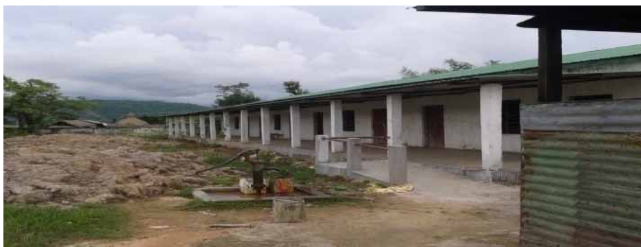
Picture-9 : Dokmoka Higher Secondary School, Karbi-Anglong, Assam – Building incomplete even after lapse of 12 months from due date of completion
