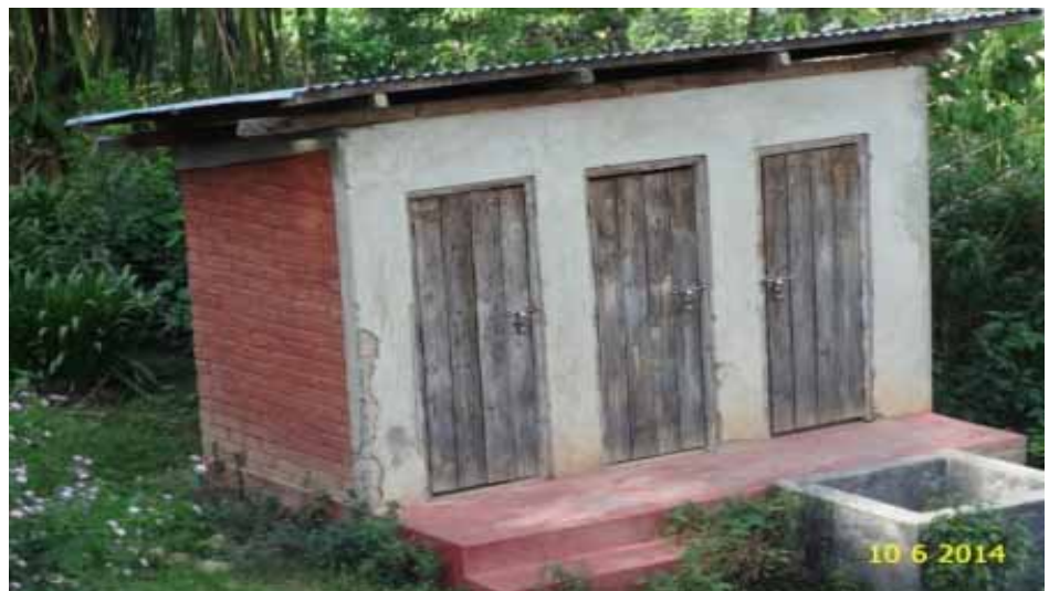
CSC without prescribed facilities at Sandangshenba Maring village under DWSM Kangpokpi Manipur
