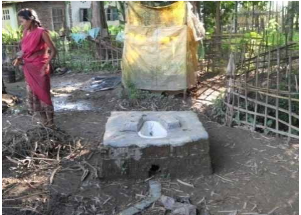
Toilet without superstructure at Rongpuria GP, Tinsukai, Assam
