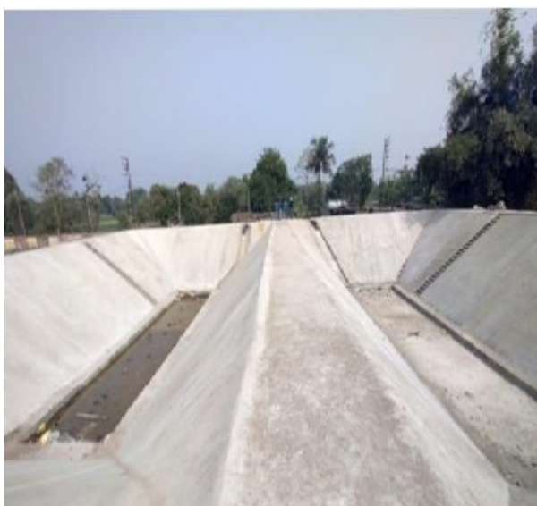
Exhibit 6.9: Partially functional oxidation pond at the STP of the Jiaganj-Azmiganj Municipality
