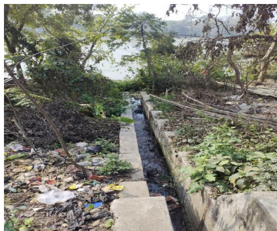
Exhibit 6.6: Untreated sewer outfall point into the Bhagirathi River, at Ward No. 07 at the Jiaganj-Azimganj Municipality
