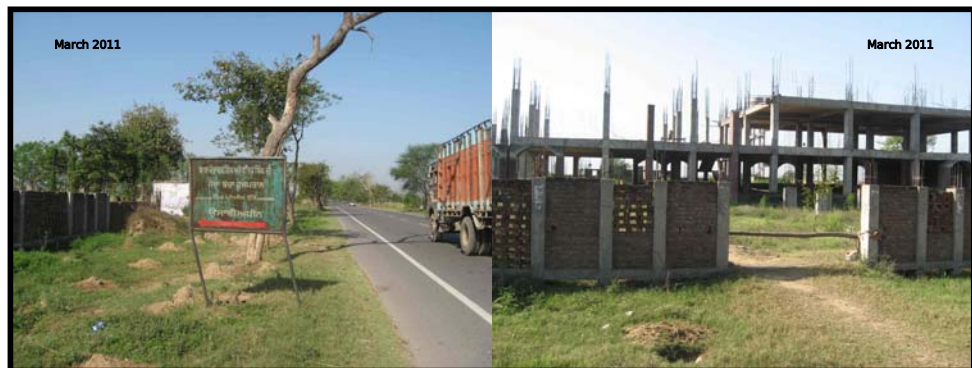
Incomplete Mother and Child Specialty Hospital building at Peerjain, Fatehgarh Sahib
