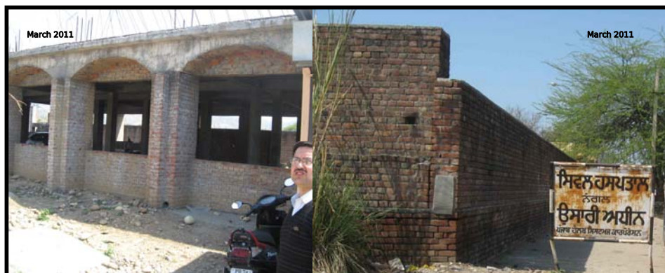
Incomplete building of Hospital at Nangal
