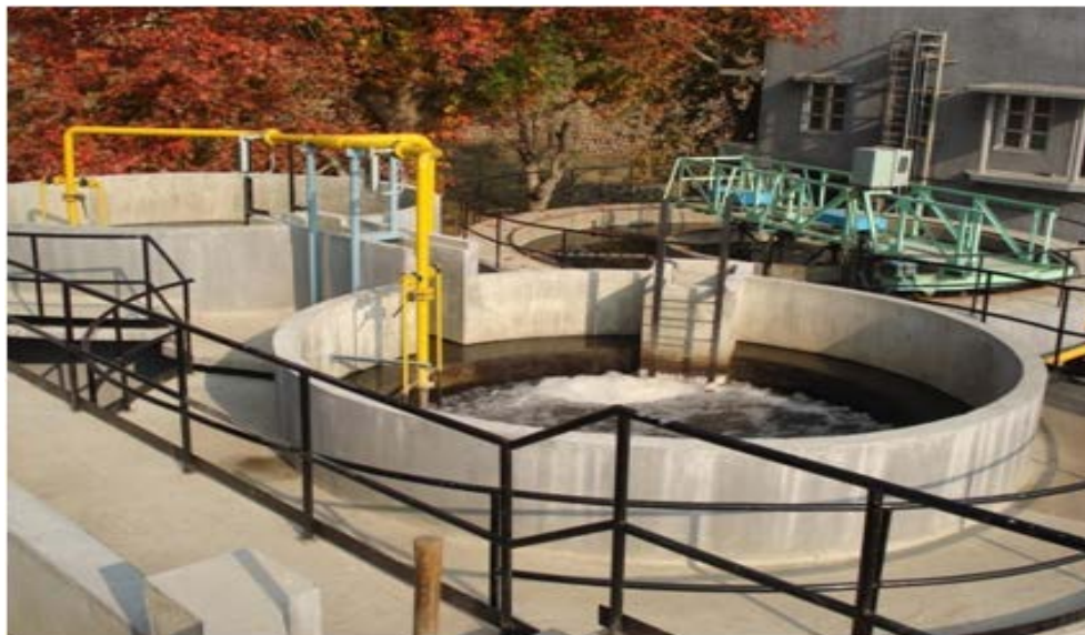
Sewerage treatment chambers of STPs without covering/roofs.
