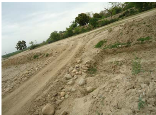
Damaged Field Drain
