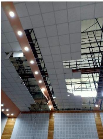
Pic 3.10: Dilapidated condition of false ceiling of the Auditorium
