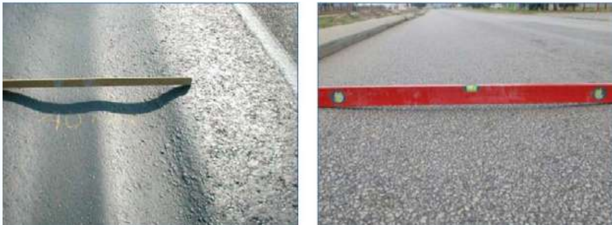
Figure 1.2: Surface depression due to rutting strain
