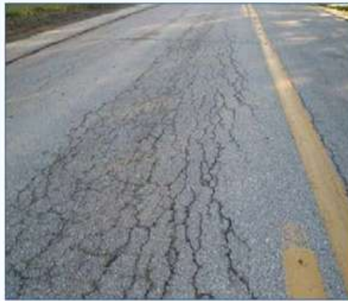
Figure 1.1: Crack of pavement due to Fatigue strain
