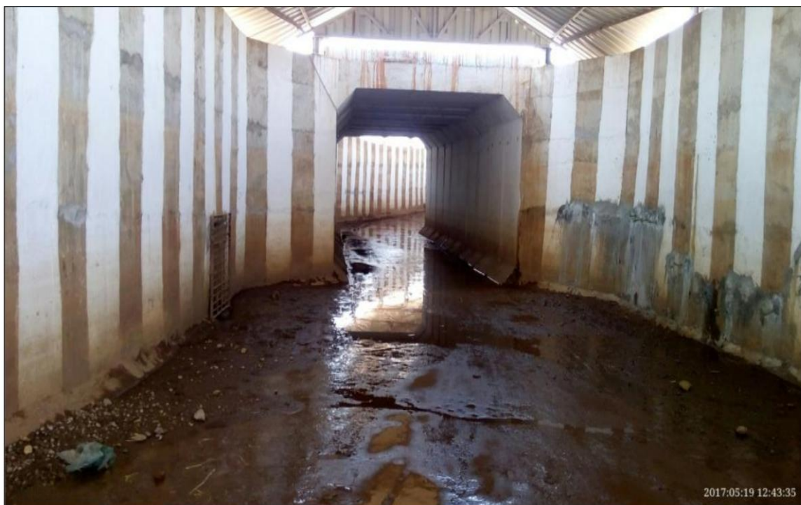
Accumulation of water in LHS due to incorrect assessment of drainage
