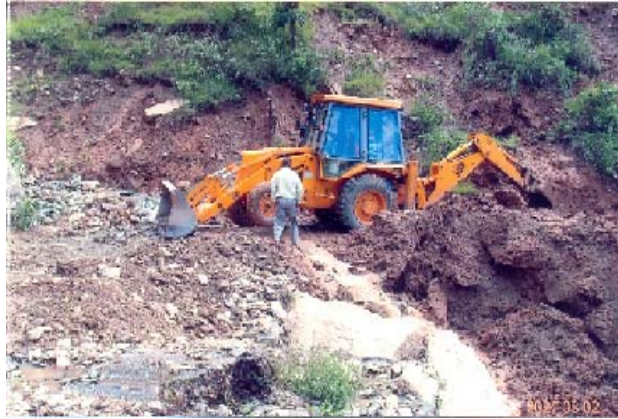
Picture: 4.1 Damaged road at km. 6.8
