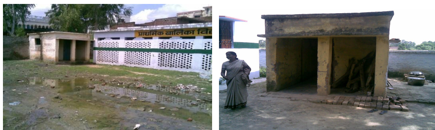
Kitchens in dilapidated condition at Rae Bareli and MDM cooked outside
