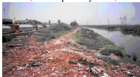
Photograph showing Jeep Track without the retaining wall (North Buckingham Canal at LS 7020m - April 2006)
