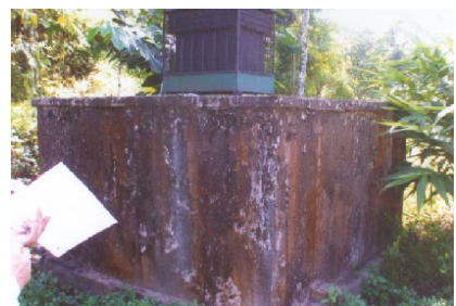
Non-maintenance of reservoir tank at Nandigaon
