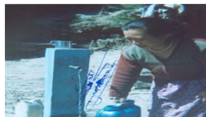
Broken tap at Phalidara (South)
