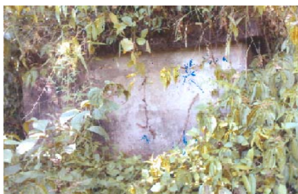
Non-maintenance of sedimentation tank at Bojoghari
