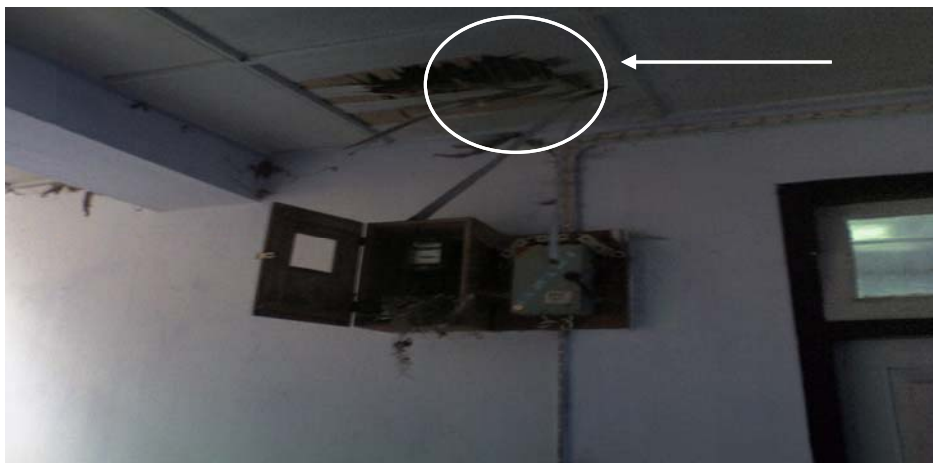
Room damaged at several places
