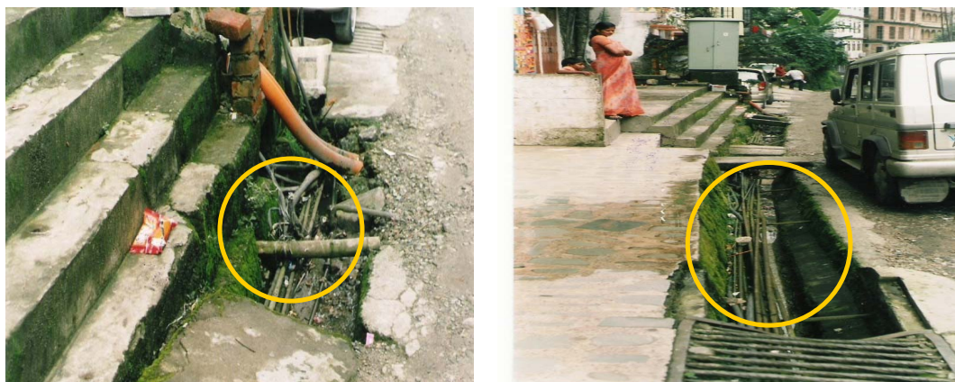
Pipelines running through drain in Tibet Road area
