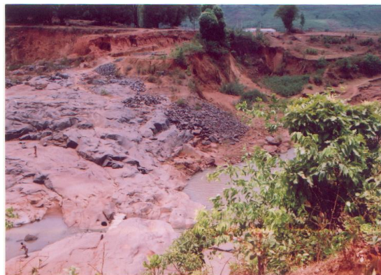
Abandoned site of the spillway of Telengiri Irrigation Project
