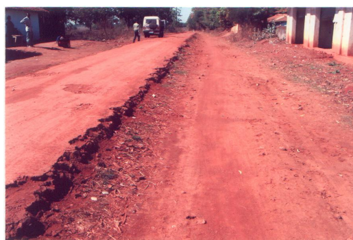
Incomplete Umerkote-Likima road
