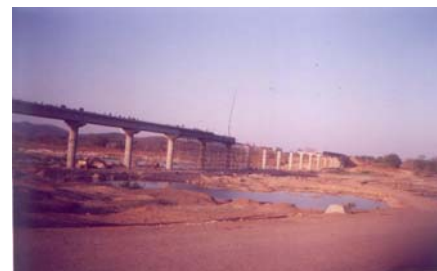
High level bridge over river IB (ITDA, Sundargarh) lying incomplete due to paucity of funds
