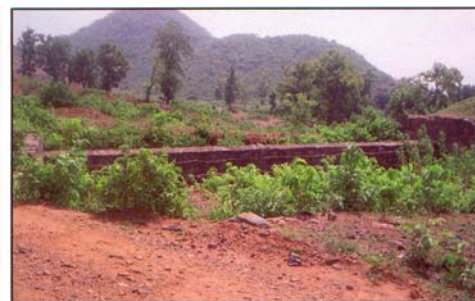
Kadaligadia MIP abandoned due to seepage in the dam
