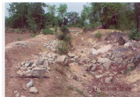
Incomplete Left Main Canal of Ghensali MIP
