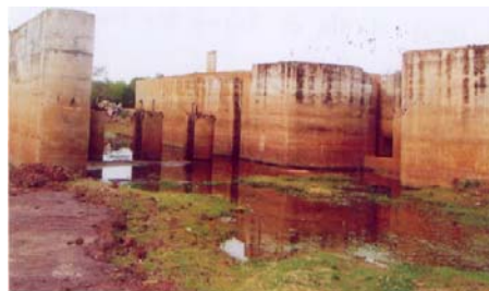
Incomplete head works of Rajua D/W
