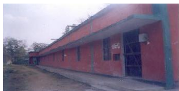
Additional ward at Anugul Jail constructed outside the perimeter wall lying idle since July 2004
