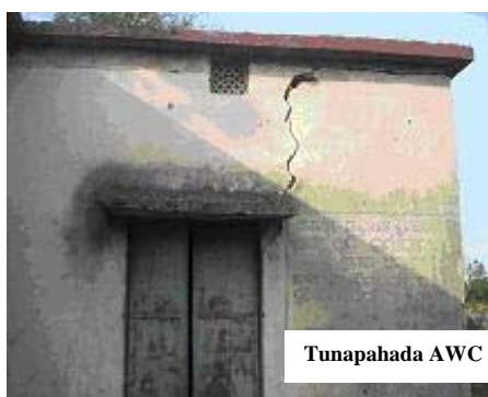
Photograph showing unsafe Anaganwadi Centre at Tunapahad
