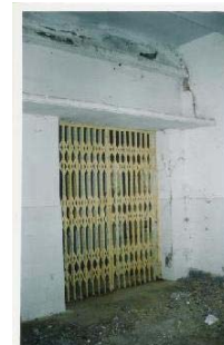
Cracks in the building of Narasinghpur Area Hospital
