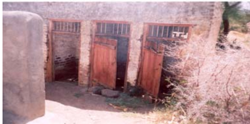
Condition of toilets and bathroom in Government Post Basic School at Jamb, District Yavatmal
