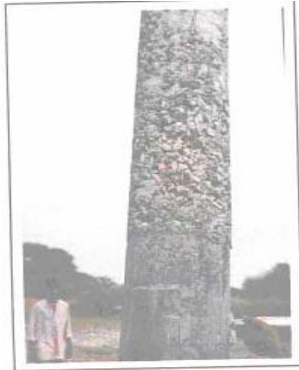
SEVERE HONEY COMBED CONCRETE IN PIERS (TYPICAL VIEW)
