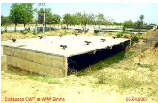
Collapsed clear water tank at water works Seehma
