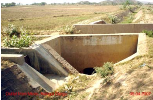
Dry outlet for water works at Nangal Dargu
