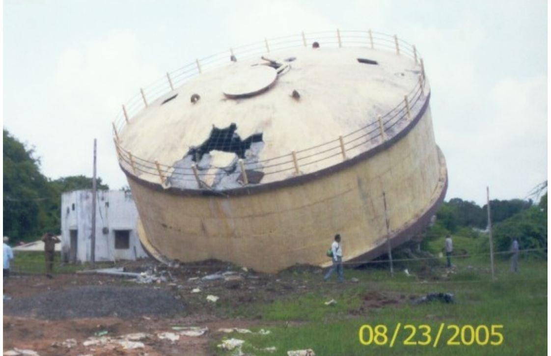
Photo showing Collapsed Elevated Storage Reservoir
