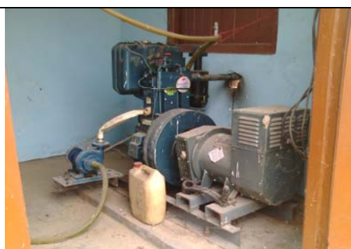
Generator lying idle for two years for want of electrical works at Bokolia CHC
