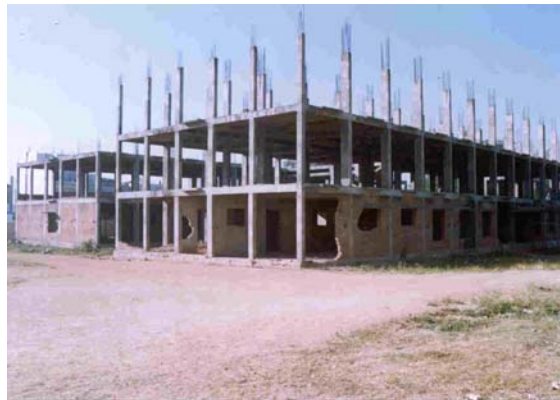
Incomplete ITI Building, Mallepally, Hyderabad
