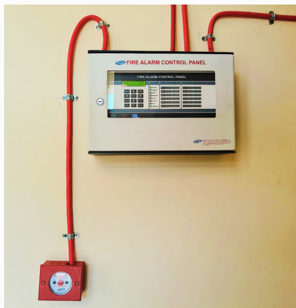
Fire Alarm safety System
