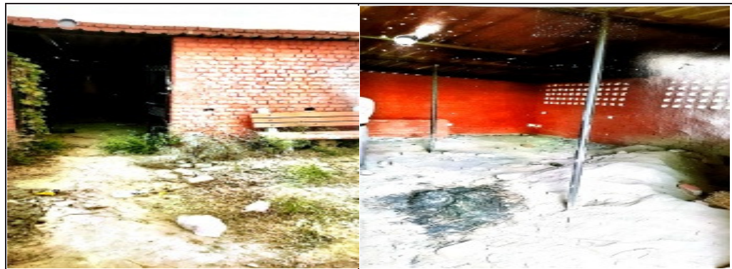
Non-functional projects (shed) for Solid Waste Management in village Joniyawas under Farukhnagar Block
