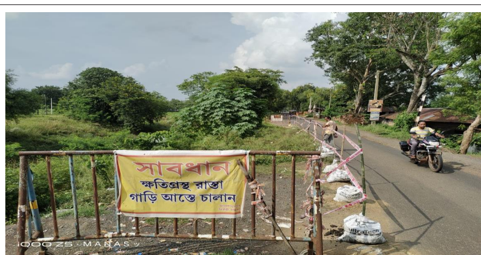
Figure 4.23: Blockage of almost half of the road due to slip faluire at the 17.050 kmp (24.08.2023)
