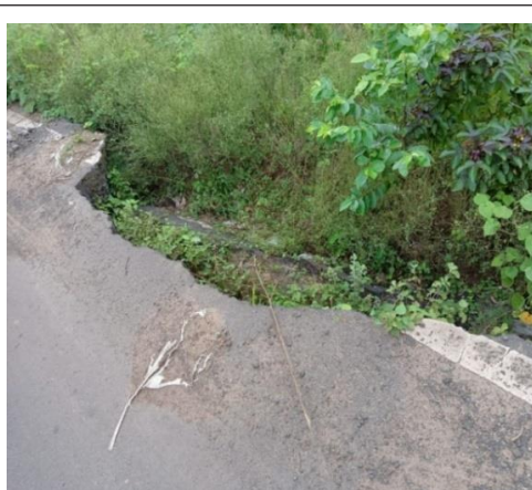
Figure 4.22: Slip faluire at 17.500 kmp (24.08.2023)
