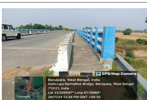
Figure 4.13: Insufficient width of footpath
