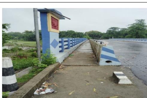
Figure 4.12: Insufficient width of footpath
