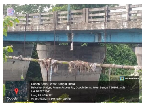
Figure 4.10: Pipeline hung with the railing of the Mora Torsha bridge at chainage 2.00 km of Coochbehar Dinhata Gitaldah Road under Cooch Behar Division (PWD)
