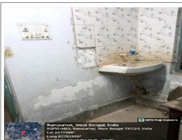
Figure 2.2: Rampurhat SAHC, Seeping walls
