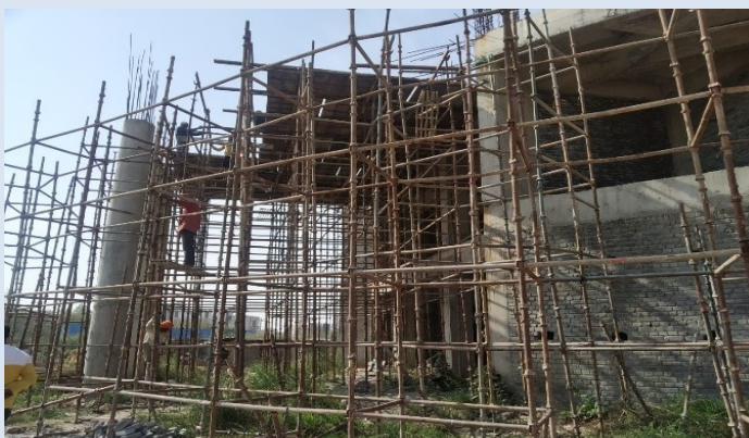
Picture 3.1: Scaffolding not covered with Tarpaulin
