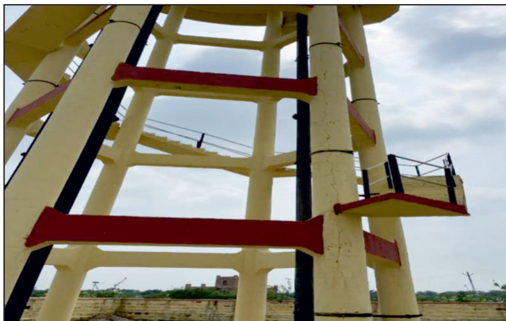
Picture 7.1: Long crack on RCC pillar of OHSR, Jatiyawas
