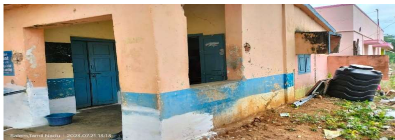
Exhibit 2.15: Materials for water supply works kept uninstalled in Saminaikenpatti AWC in Omalur Block of Salem district
