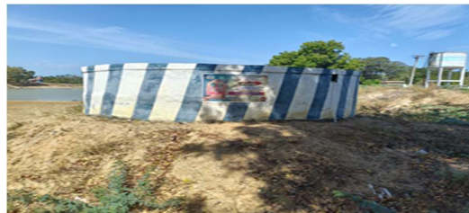
Exhibit 2.2: Open well at Thinaikulam VP not used
