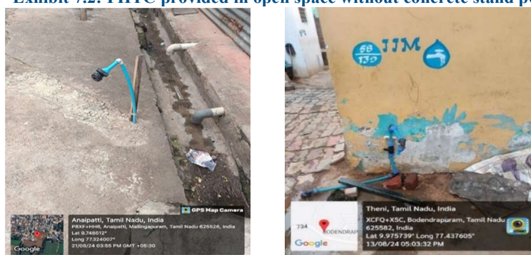
Exhibit 7.2: FHTC provided in open space without concrete stand post
